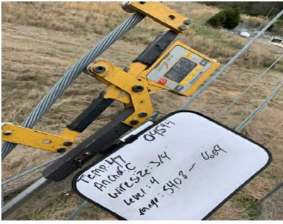
Anchor A Guy Level 1
