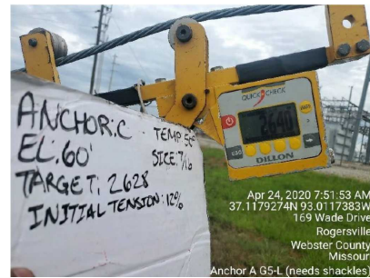
Anchor A Guy Level 2
